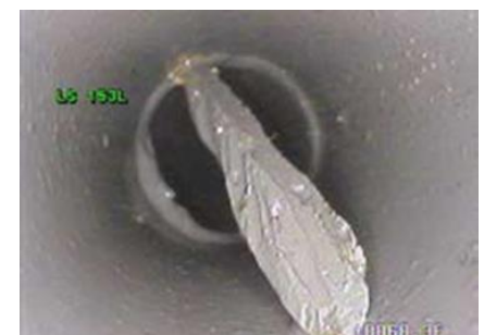
Obstructed Boiler Tube
